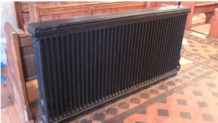
Photograph of the early radiators dating from the 1905 heating system
